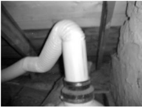
Dryer vent in Attic??
