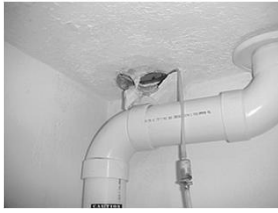
Caused Leak Through Ceiling
